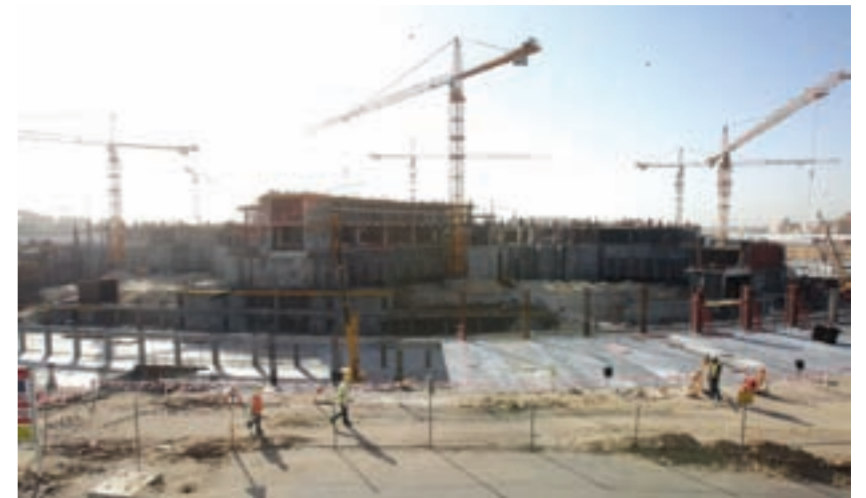
FILE - Seen here is the construction site for the Jaber Hospital, expected to be one of the largest medical institutes in the region, located at South Surra, Dec. 2, 2011. (Al Watan)
